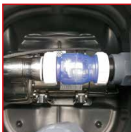
Check valve and sewage water pump
